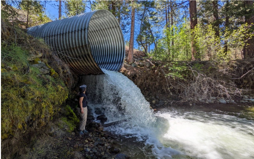
Cold water pouring out of a perched culvert during late summer during a historic drought, 2022. Coho Salmon listed under the Endangered Species Act are waiting below the culvert to move upstream to historical rearing habitats. This project would replace the culvert with a bridge- providing year-round access to high-quality upstream habitats.
